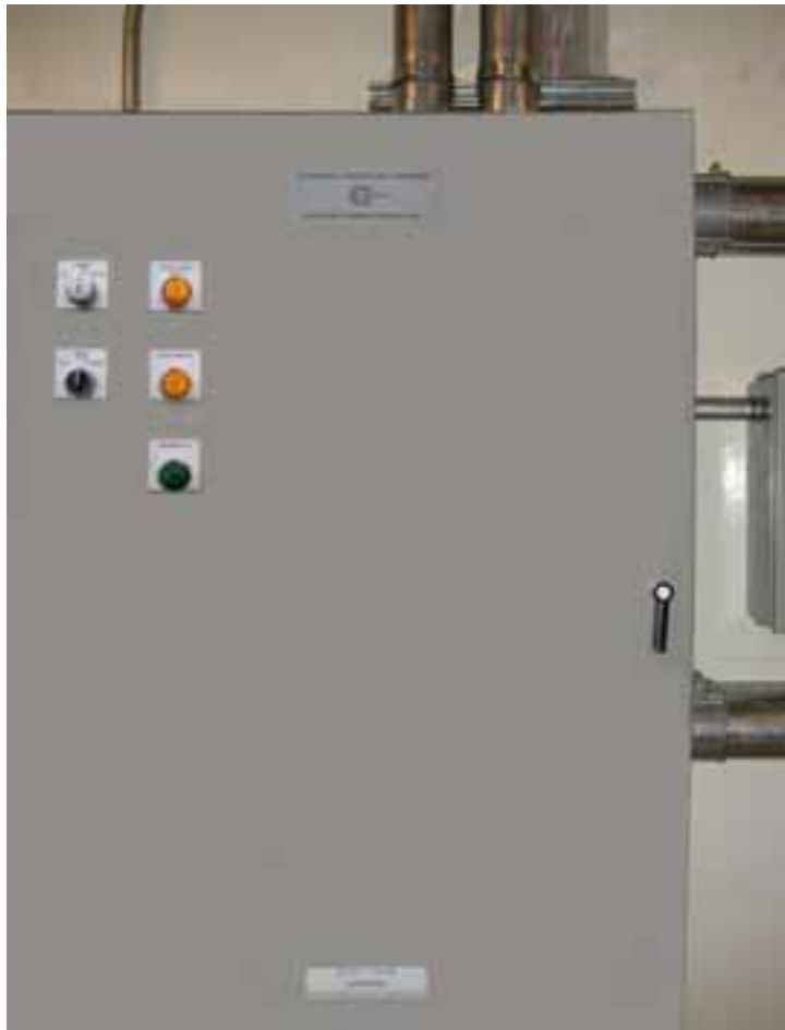
Figure 5. Typical Indoor DMC Installation
